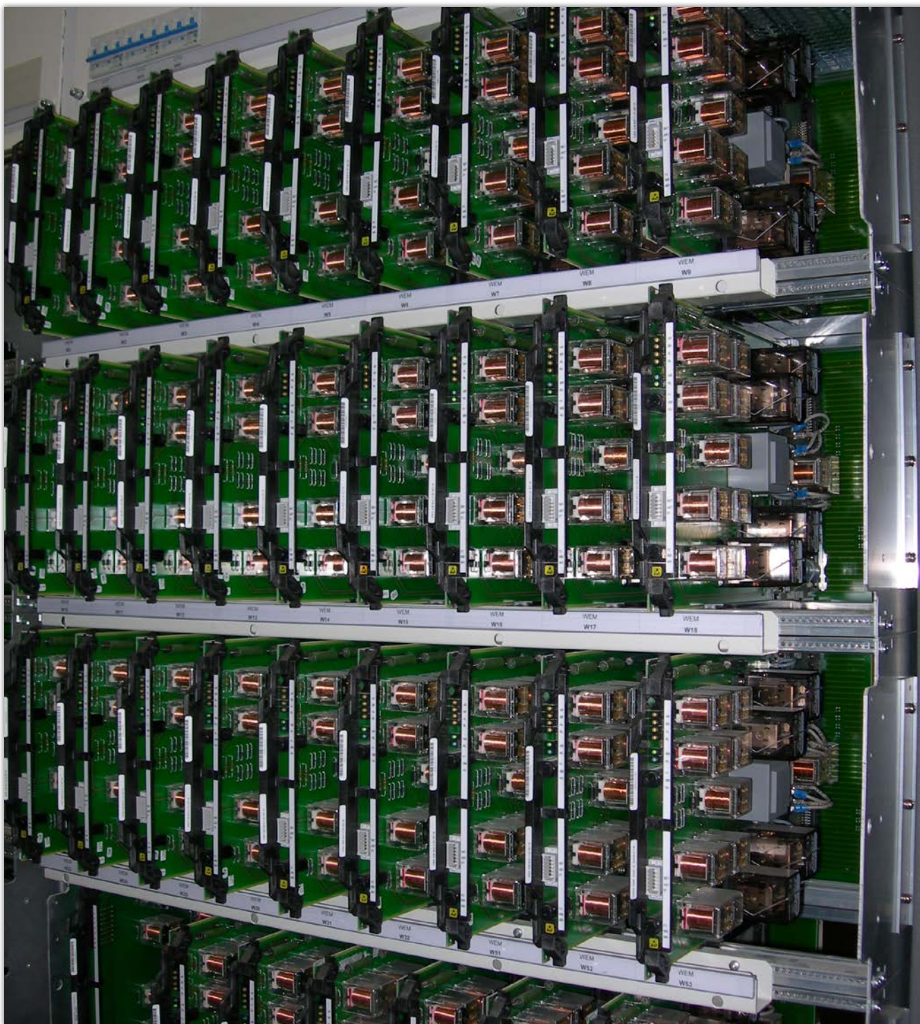
Figure 89: Relay control devices in an electronic interlocking of type ELEKTRA
