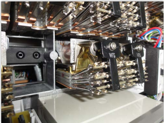
Figure 32: K50 relay as part of a relay group
