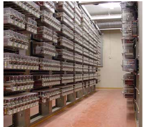
B-relais rekken in relaisruimte Bron ProRail
